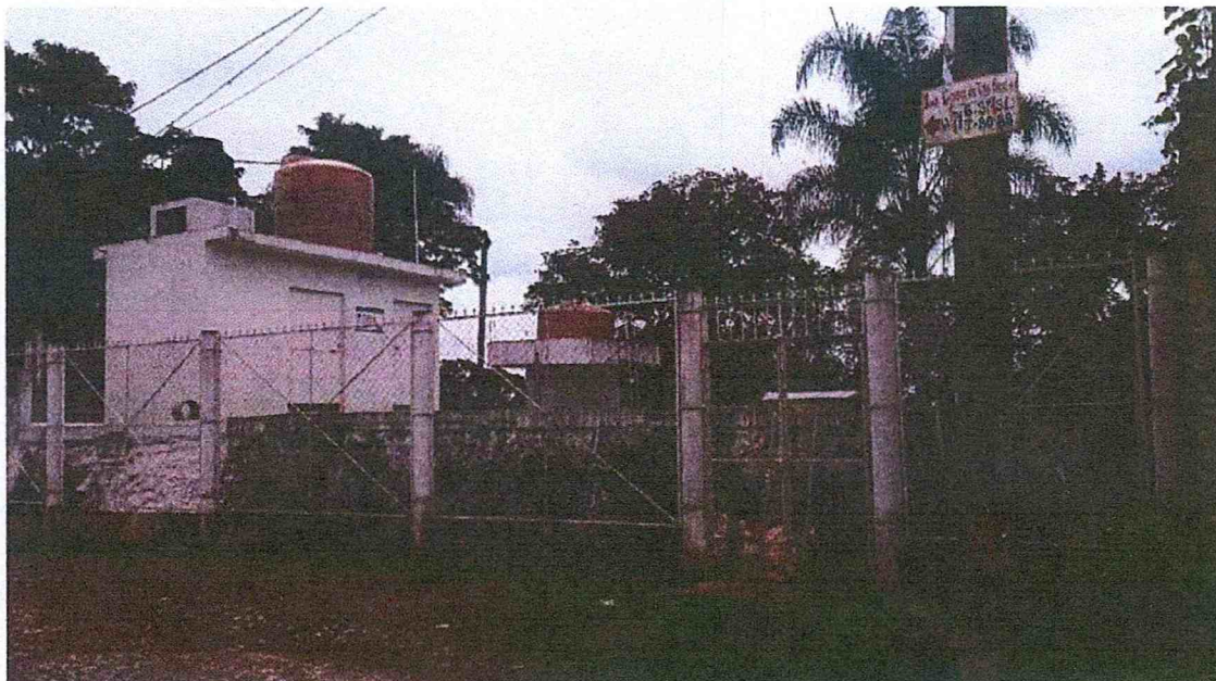
TANQUE TOXPAN H007
